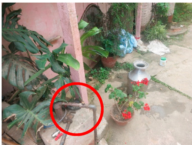
Fig. 5. Condition of the main valve.
